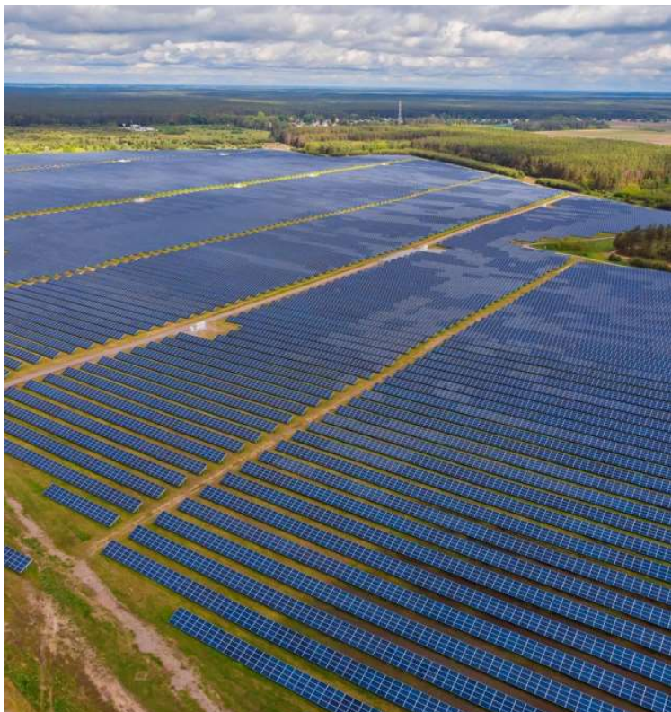
Representative ground-mounted solar imagery
